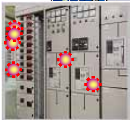
Motor Control Center
